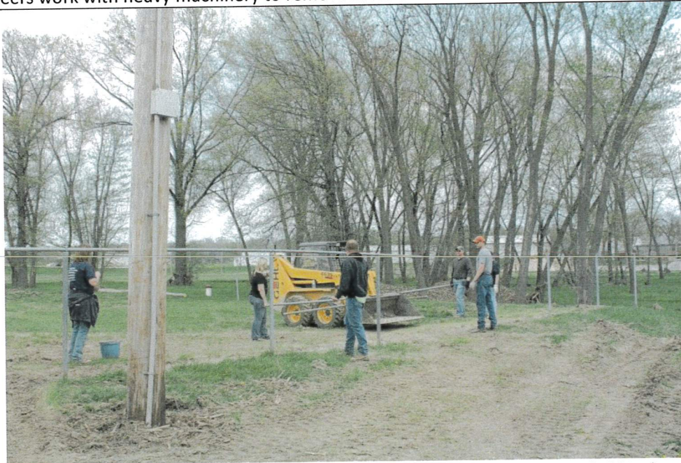
Volunteers work to rebuild fence that was destroyed by the river current. Much of the field is destroyed each year with debris and dumpsters, trash cans, and septic tanks being spilled into the Weldon/Grand River. (2013)
