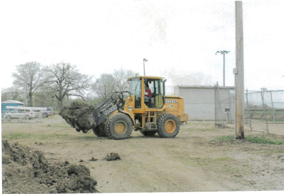
Volunteers work with heavy machinery to remove silt and debris from the ball field complex (2013)
