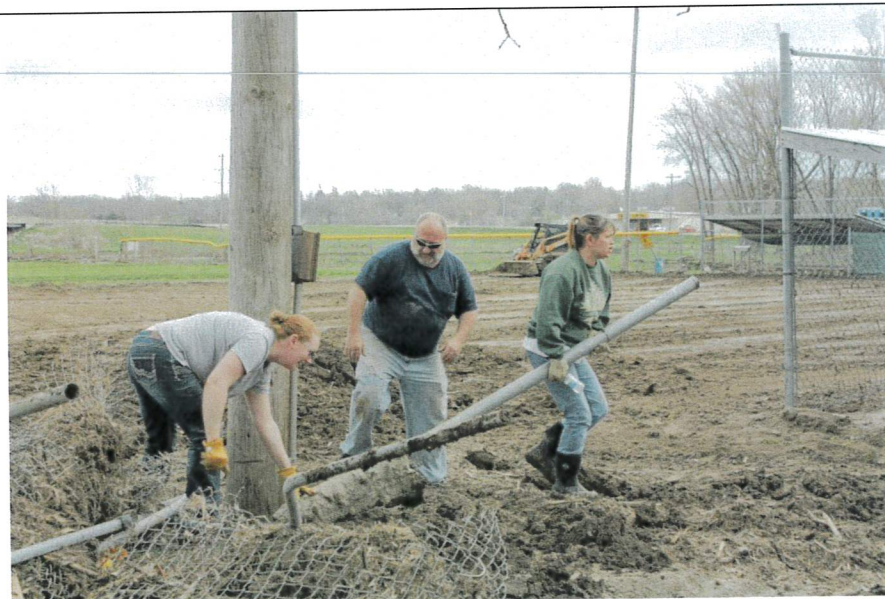
Volunteers work to fix fence after river currents cause damage to the ball fields. (2013)
